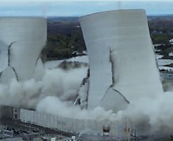
KEEP IT SIMPLE: Pangaea CEO Ed Coll (left) says the secret to success is not complicated. Above, demolition of the cooling towers at the Brayton Point site in Massachusetts
